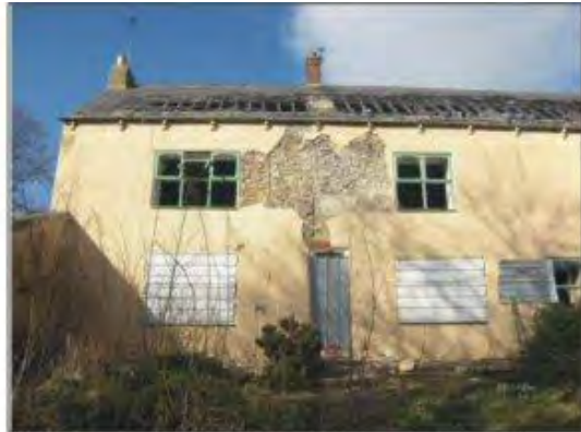
West part of Gore Hall farmhouse, south frontage, showing masonry join (above door)
