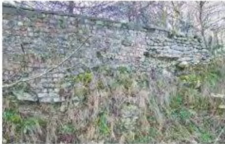
Brick and stone boundary wall between Wingate Farm and quarry to the east.
