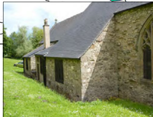
Exterior view of the Thornley Porch at St. Helen's, Kelloe, from the NW. Originally a chantry chapel supported by income from land in Thornley and Kelloe.
