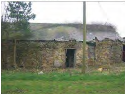
The west end of the north elevation of the detached NE range.
