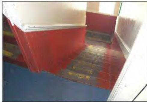
Stairs to first floor in schoolroom block, with original wall panelling and handrail.
