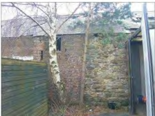
Detail in the central part of the north wall of the NE range, showing stone and brick masonry, infilled vent, etc.
